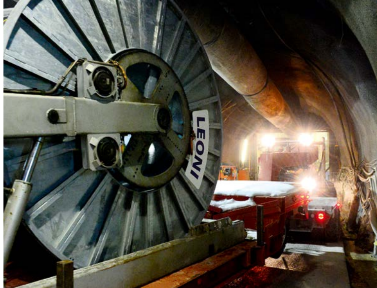
High-precision transportation of cable reel and laying machine, deep in the mountain.
